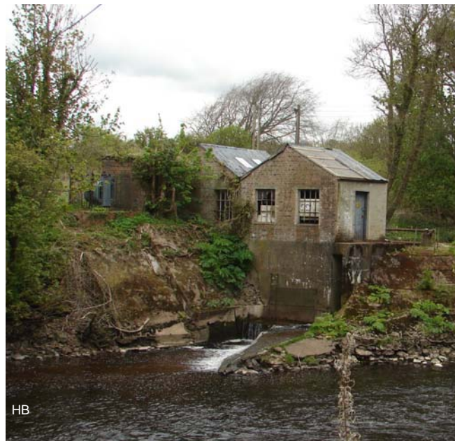
Milton Mill is now used as storage and the drop of 15 feet of water was used for a 58 kW Kaplan turbine variable pitch (made by Boving and installed in about 1935) coupled to a DC generator to supply electrical energy to the mine. A regulator controlled the pitch of the blades to match the load.
