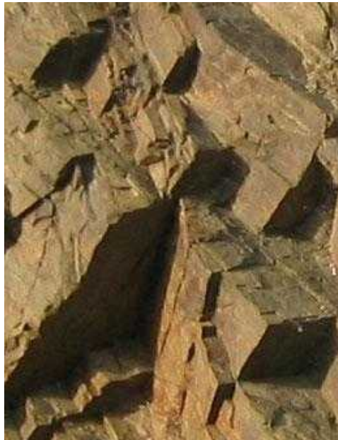
Figure 4. Detail of the rock face area that is used to demonstrate the method. Refer to Figure 2 for the position. The dimension of the area is about 1.5 x 2.0 meters.
