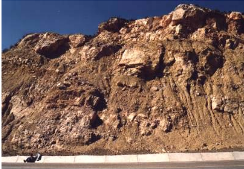
Fig. 9. Photo showing instable slope of example I.
