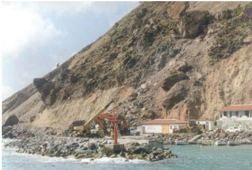
Fig. 14. Landslide in the harbour of Fort Bay of February 1997
