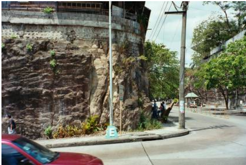
Fig. 15. Failing slope in Manila
