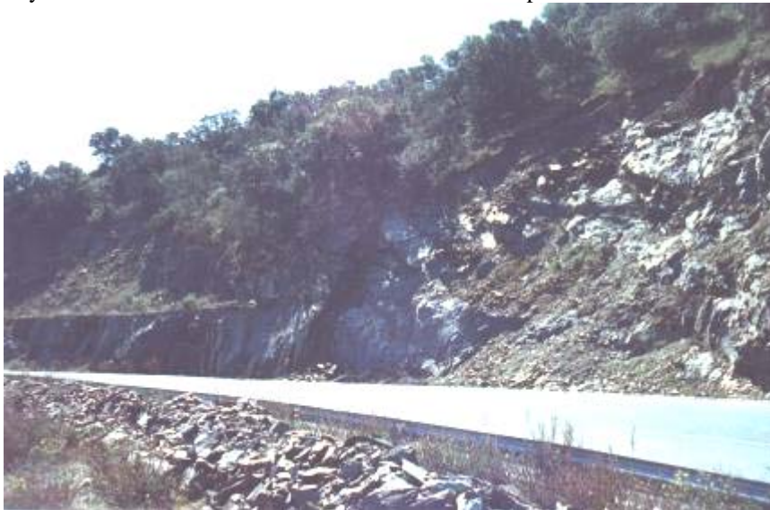
Fig. 12. Example III. The slope in April 1995 after the main failure of April 1992 and the partial failure of the top part of the slope (the terrace on the left is the old road).
