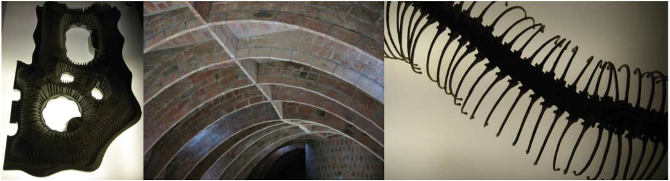
Figure 3. The roof structure of Casa Milà: overview maquette, detail of actual structure, skeleton of a snake.
